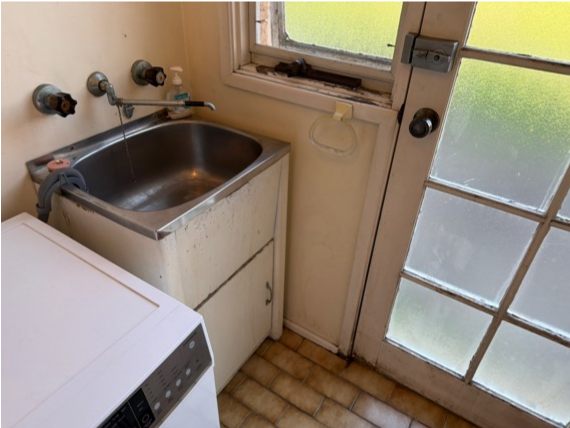
The laundry tub displays moderate level wear, cabinetry is heavily worn and architraves require remedial works.
