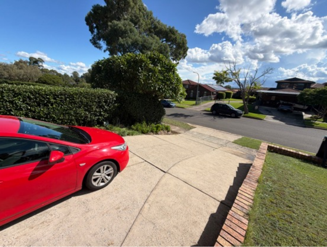
Isolated sections of exterior concrete displays typical shrinkage cracks and undulations - consistent with age.
