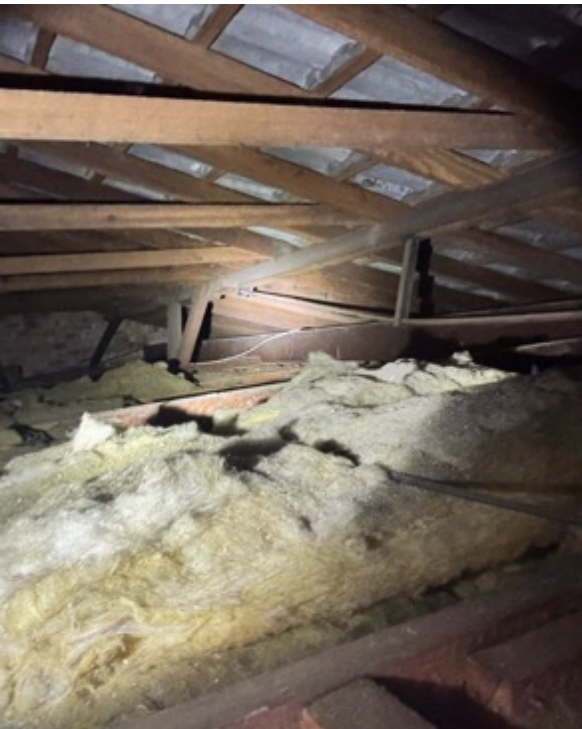
Maintain regular pest control by means of baits, sprays and monitoring to prevent pest attack within the roof space.
