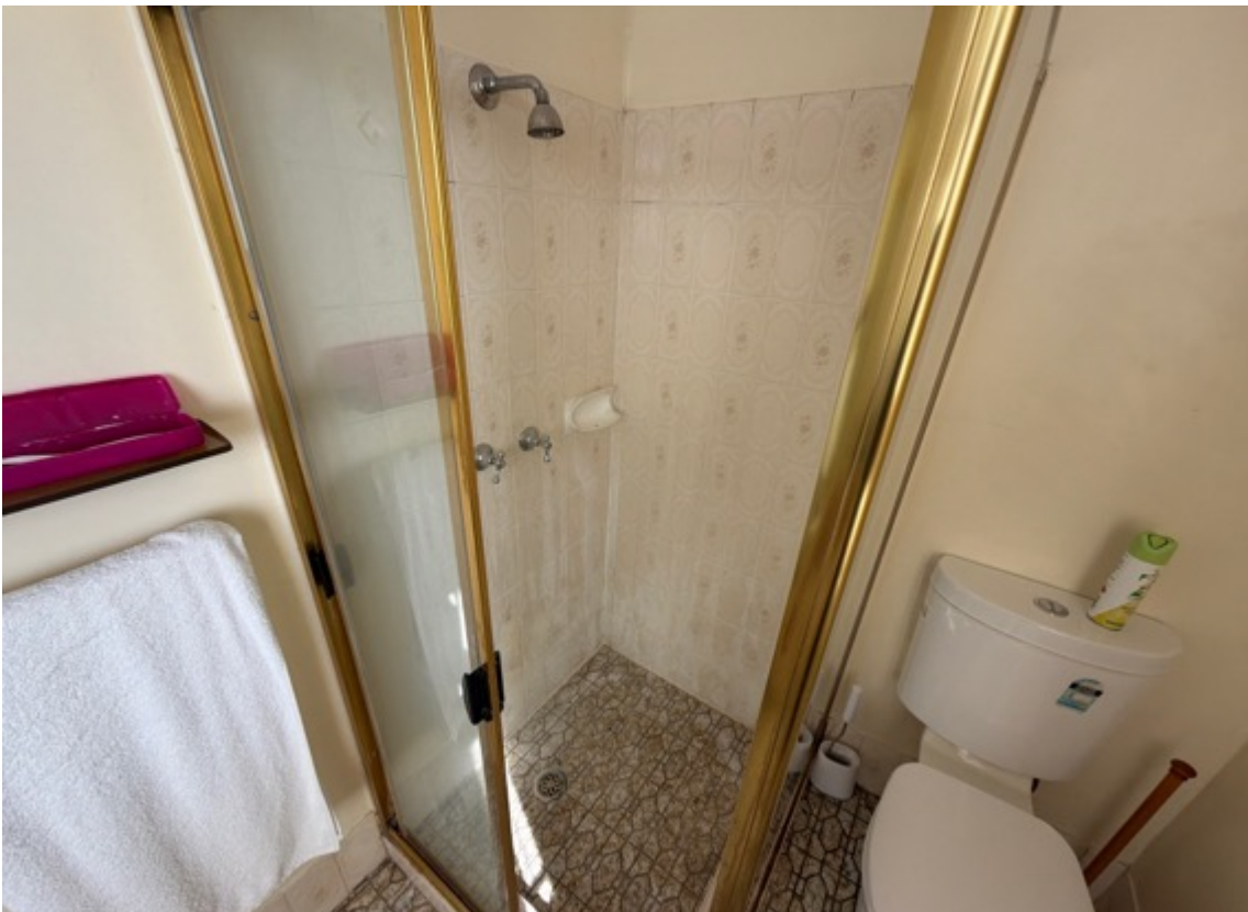
Water pressure tested, is sufficient - tile grout and silicone is darkened - reapplication is required.
