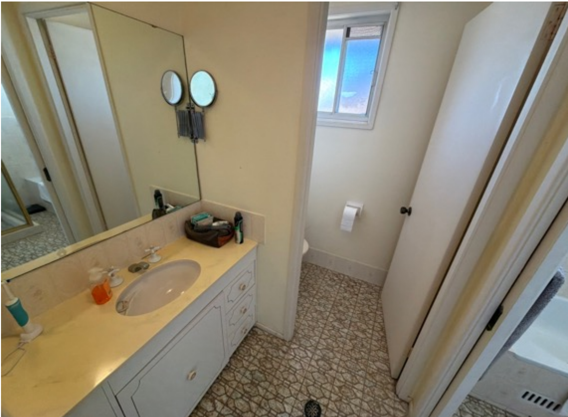
The first floor common bathroom area water services tested, functioned at the time of inspection - renovations are required due to the age.
