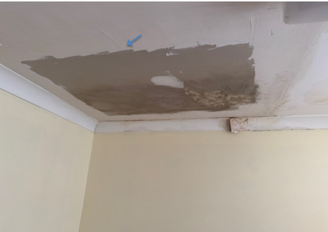
Past water staining is visible, plasterboard and cornices will require replacing in the front mid section bedroom area.
