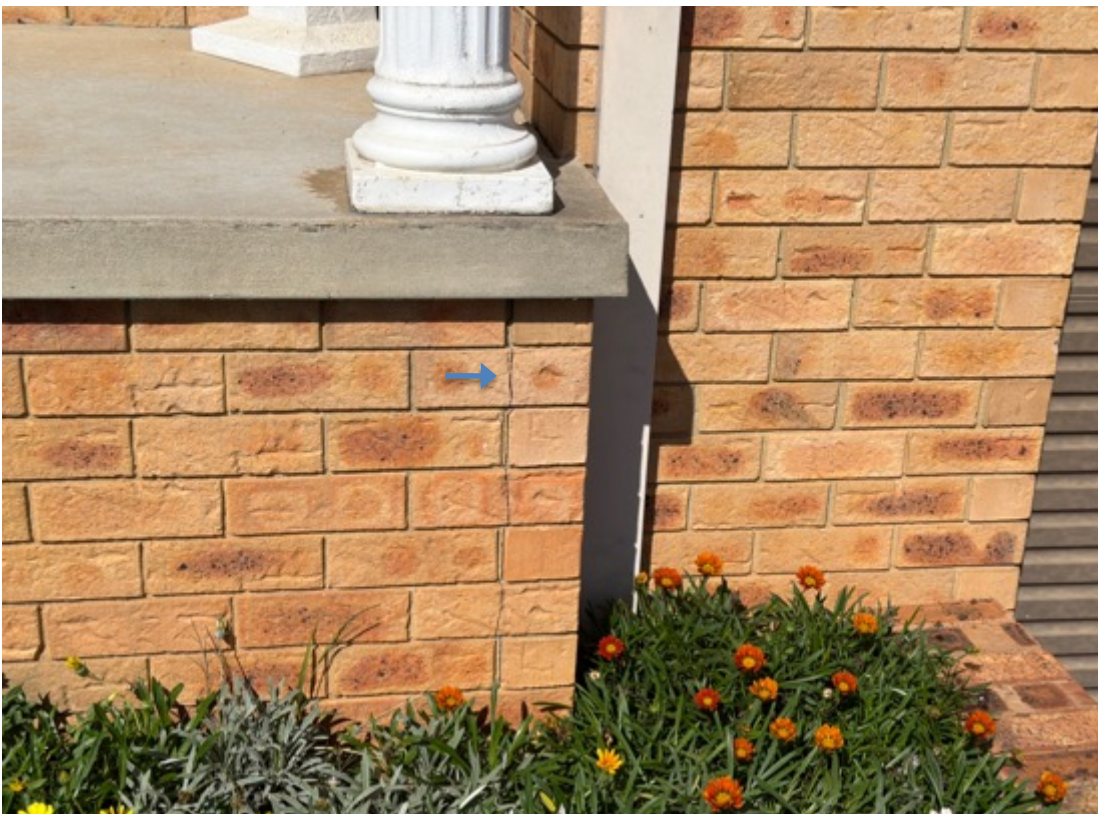
Exterior brickwork displays category one - two cracking (front mid section example above.)
