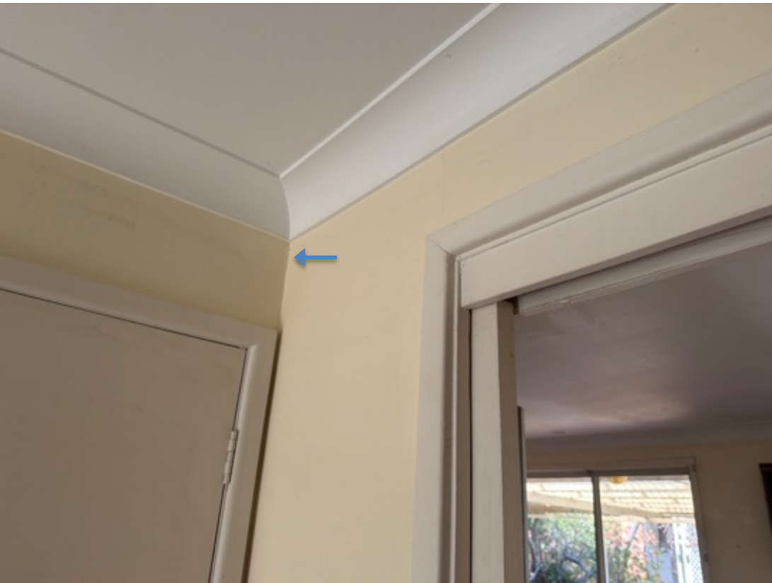
Sections of plasterboard and cornices are cracking (example above the kitchen entry cavity slider.)
