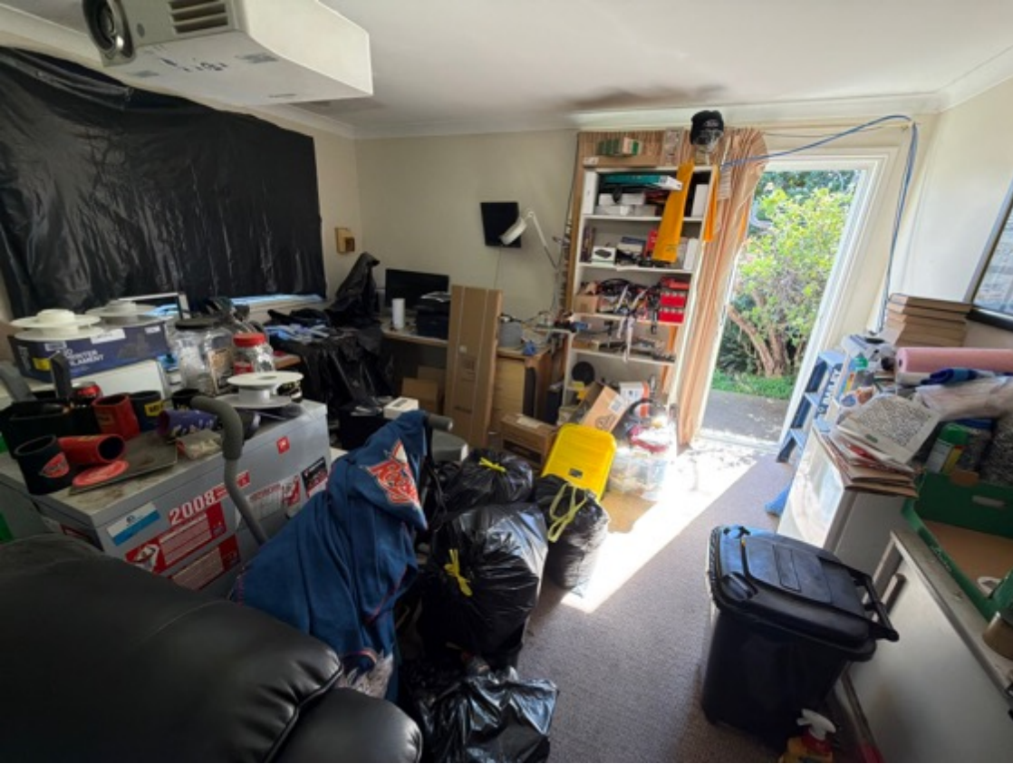
The granny flat interior is in serviceable condition, renovations are required due to the age.
