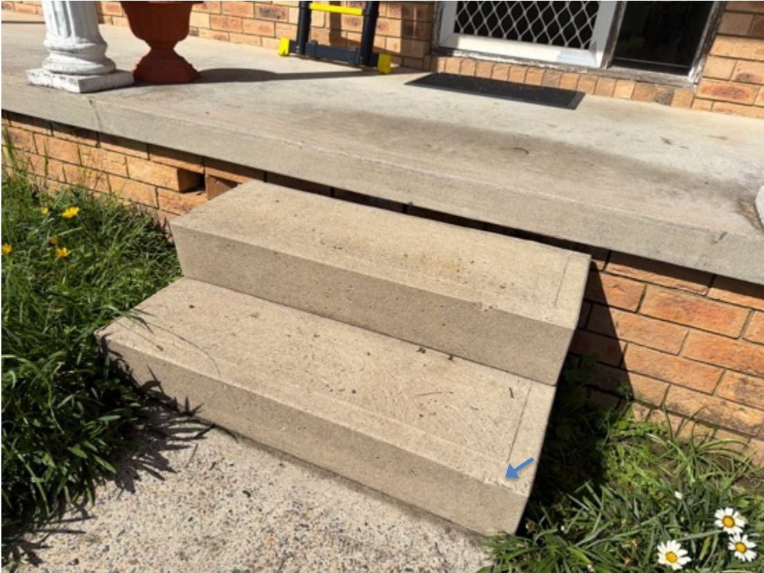
Front patio steps require remedial works.
