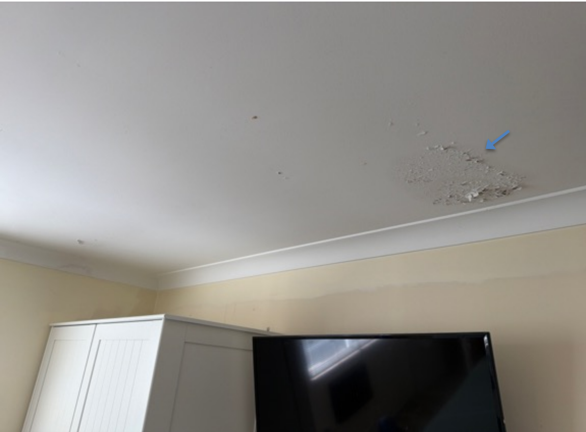
Ceiling paint is peeling, a fresh coat of paint is required.
