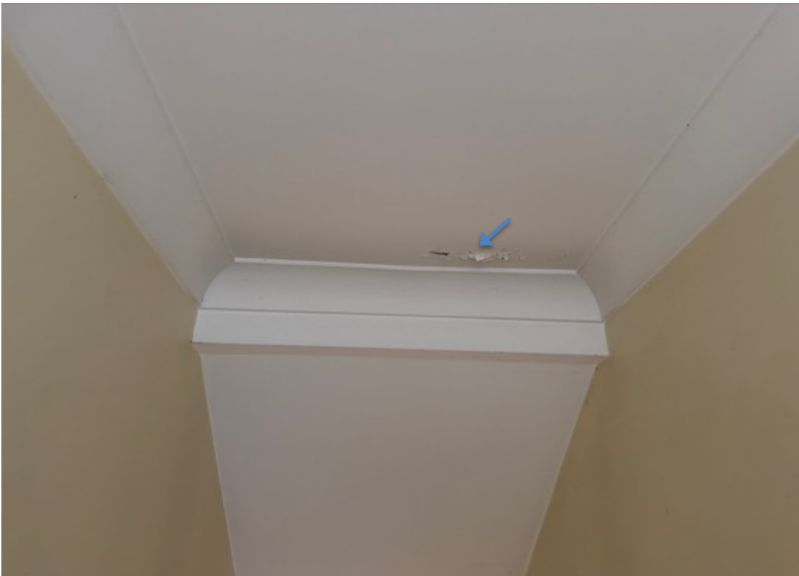
Top of bedroom hallway (above staircase) plasterboard has water damage here.
