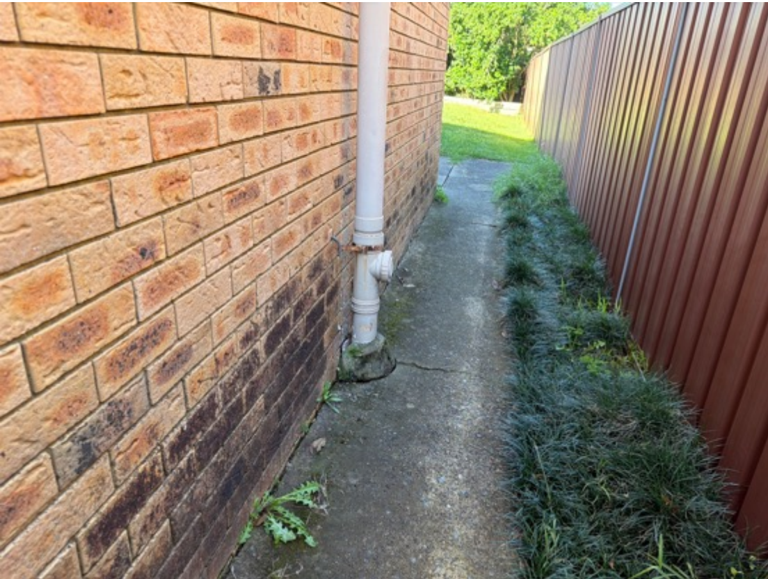
Right side footpath has subsidence.
