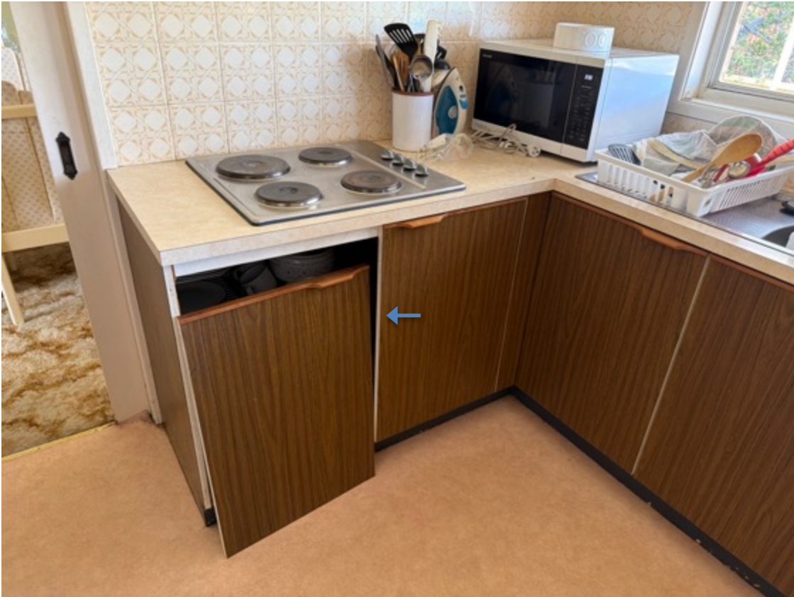
Cabinetry displays moderate level wear, sections of cabinets have come loose.
