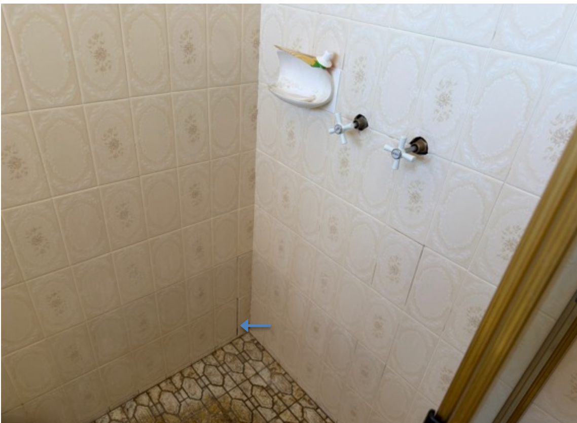
Shower wall tiles are drummy and hardware requires replacing.
