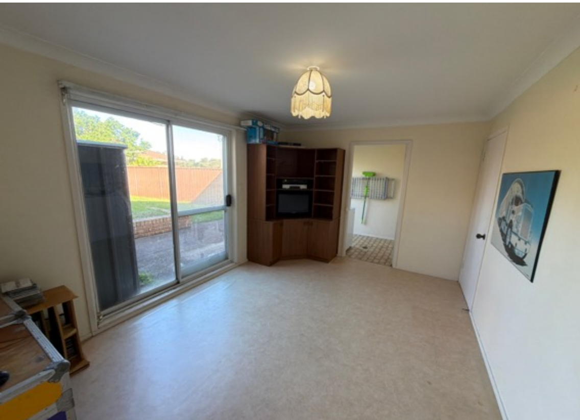
Plasterboard and cornices display imperfections.
