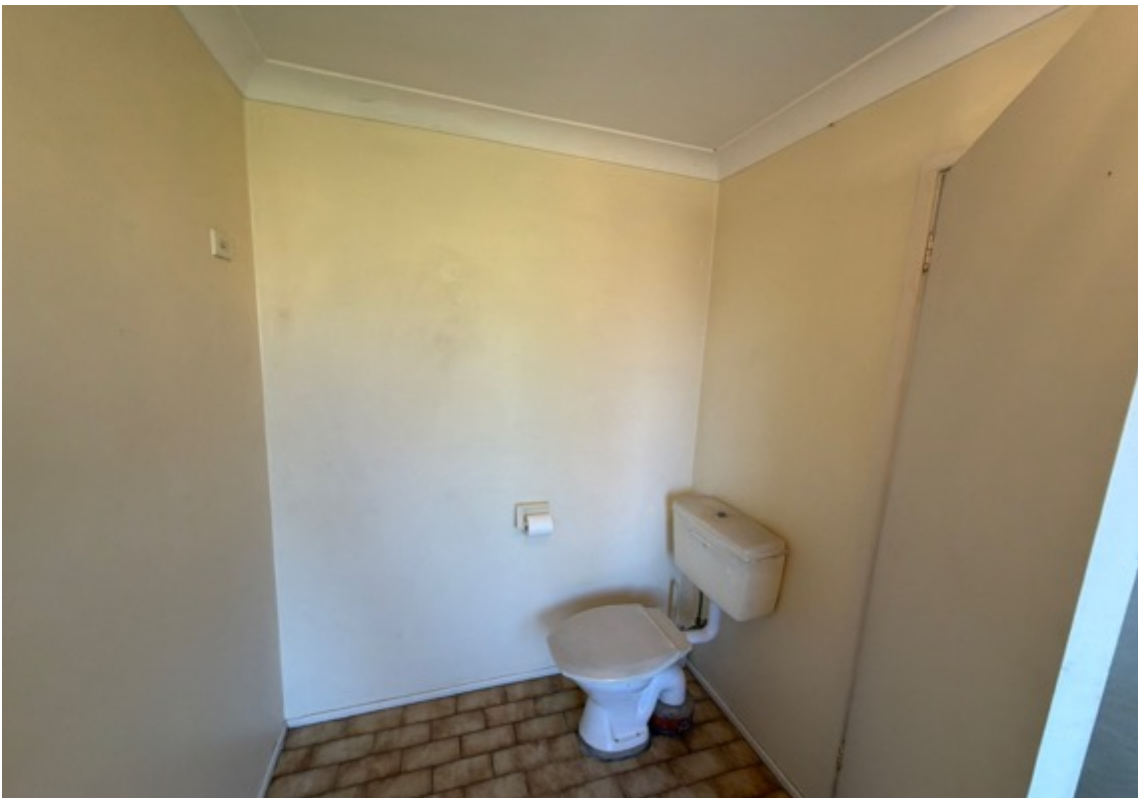
The toilet tested, functioned at the time of inspection - plasterboard and cornices are cracking.
