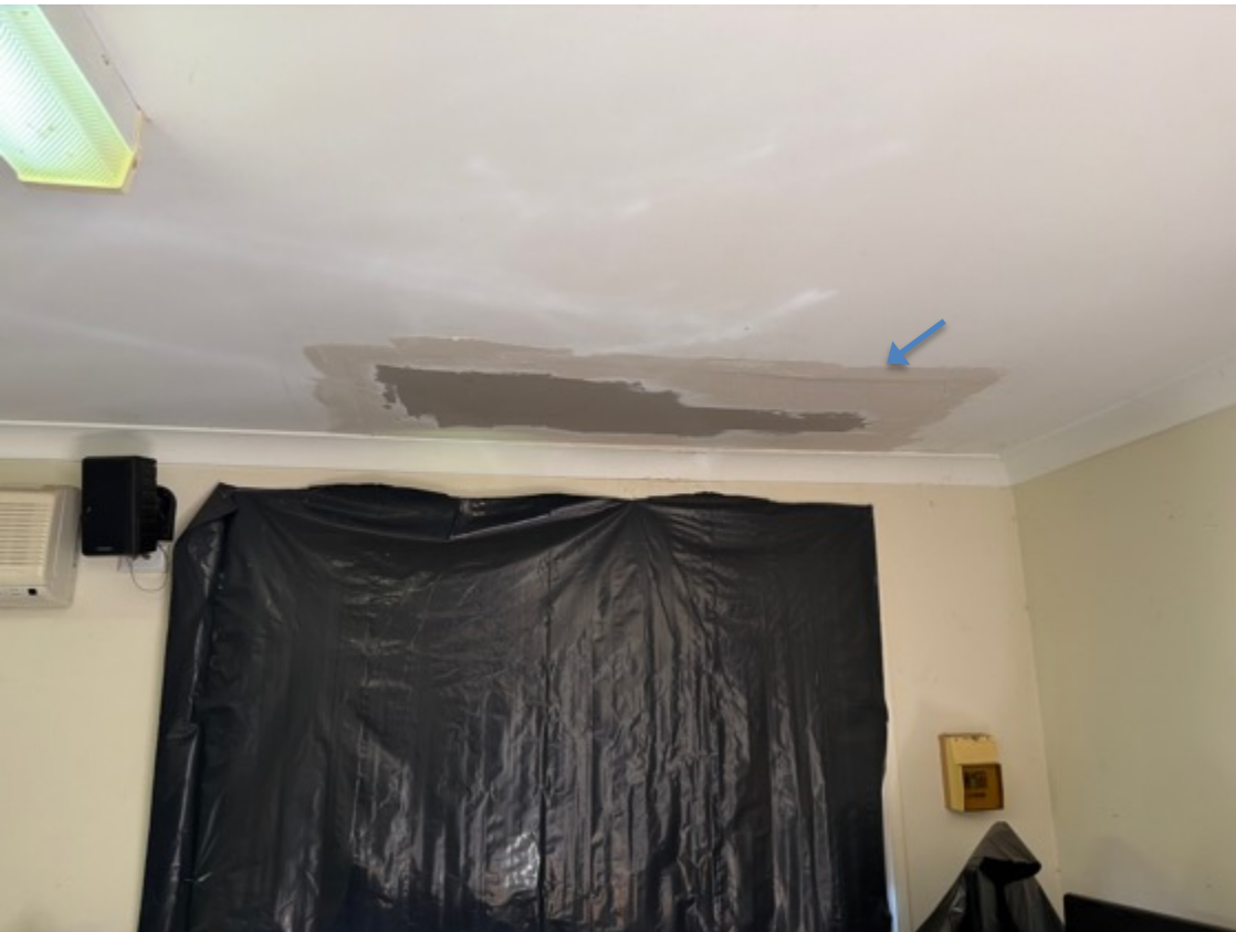
Painting works are incomplete and plasterboard has patches here.
