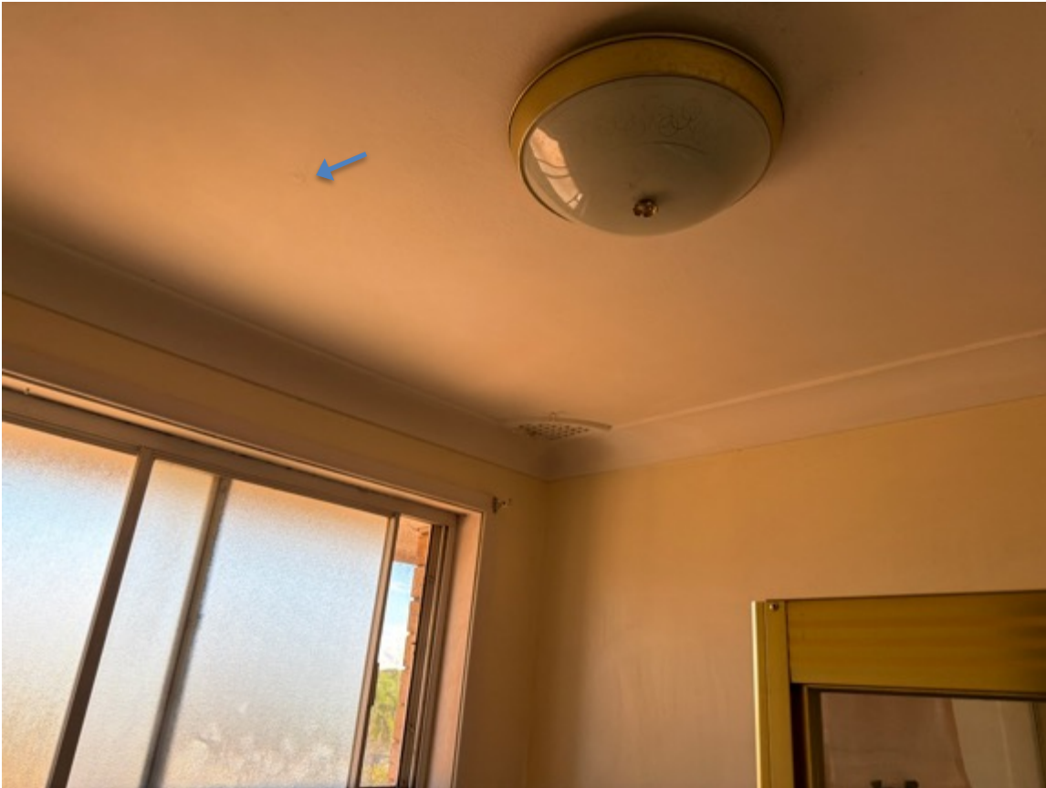
Ceiling paint is peeling, a fresh coat of paint is recommended.
