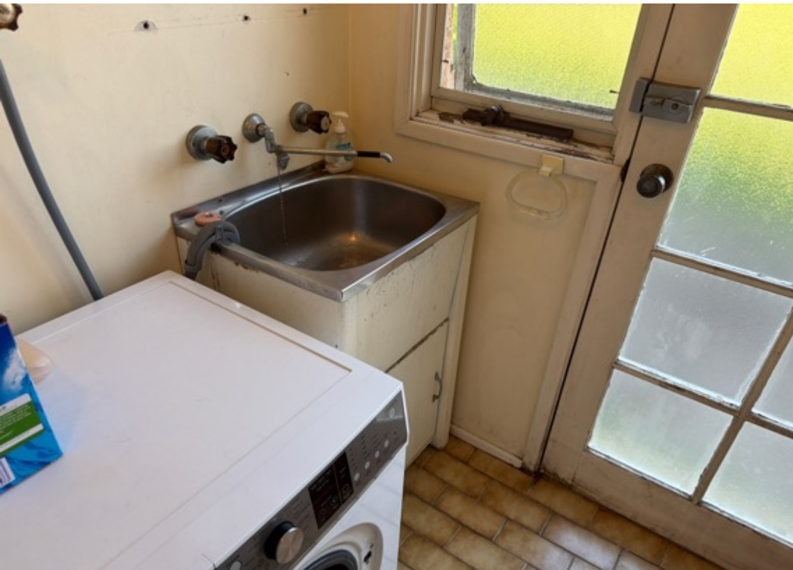
Water pressure tested, is sufficient.
