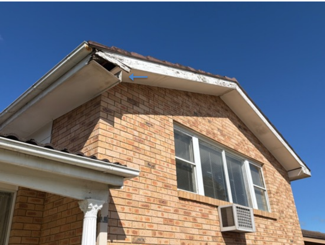
Exterior timber displays heavy level weathering - rotten, consistent with age.
