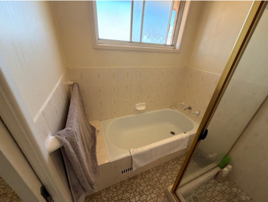
Hot and cold water services tested, functioned at the time of inspection.
