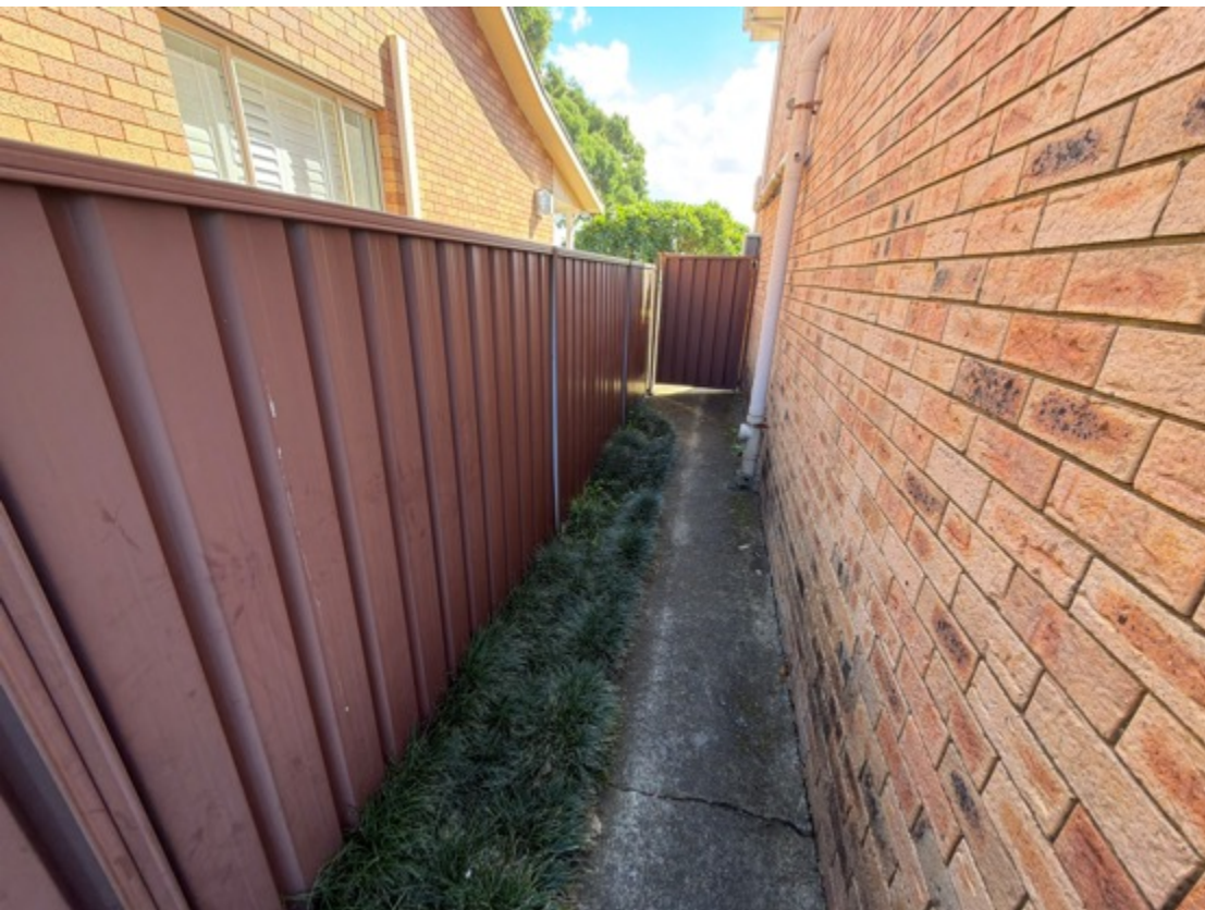
Site fences are in serviceable condition, have sections of damage and are leaning.
