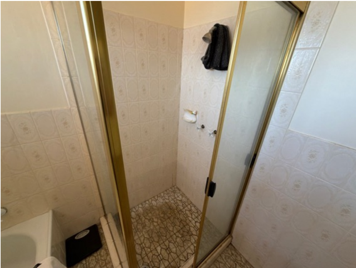
Water pressure tested, is sufficient.
