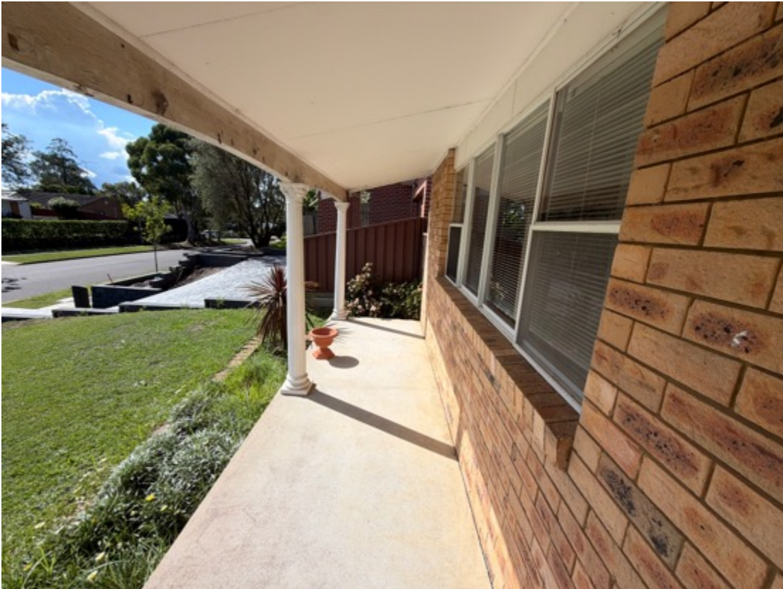
Exterior surfaces are moderately paint blemished, a fresh coat of paint is recommended on each elevation.
