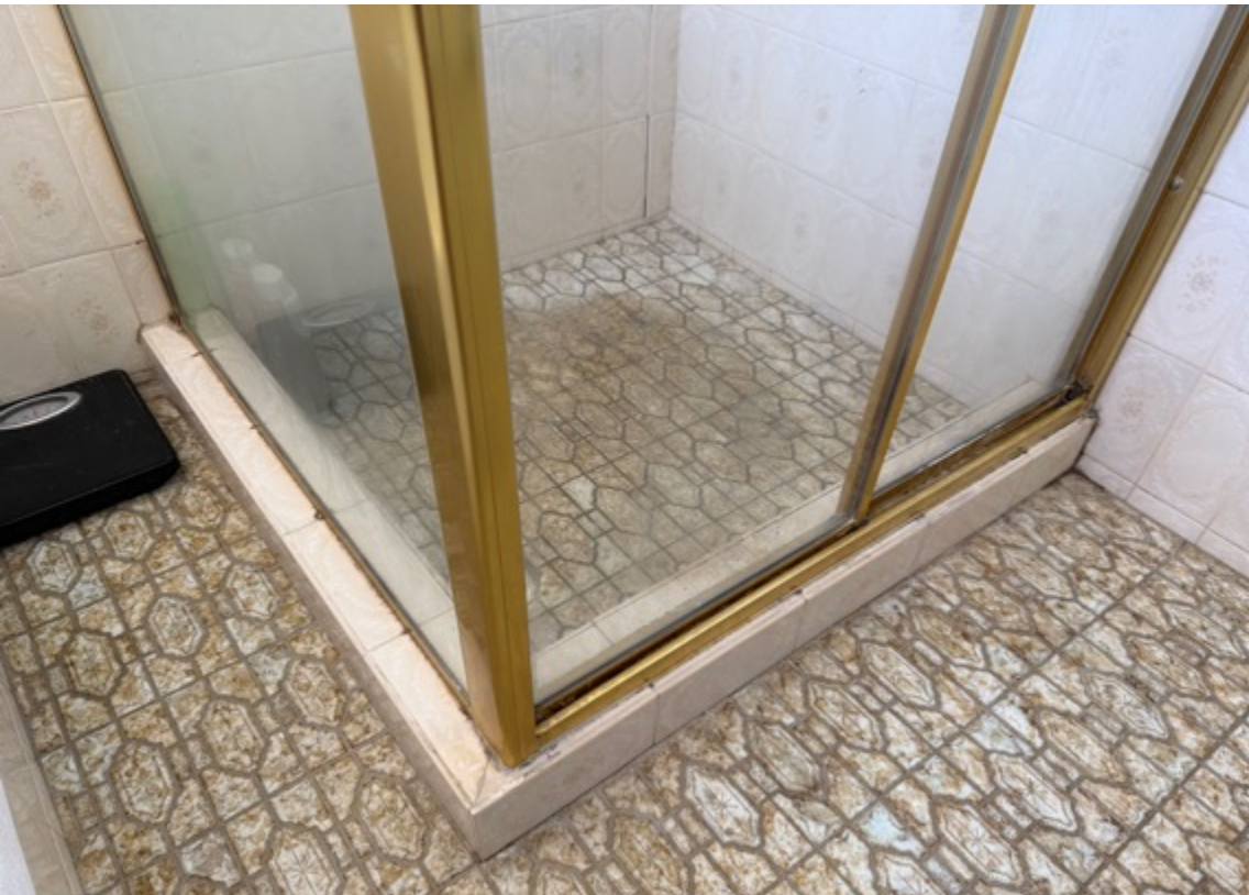
Sections of tiles are cracked, and grout - silicone requires reapplication.
